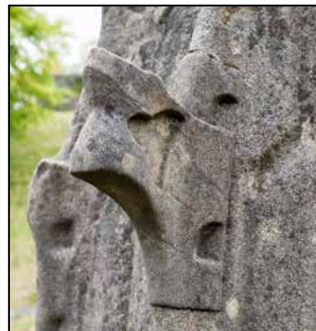
Differential weathering between the pinnacle and an earlier repair using an unknown stone.
