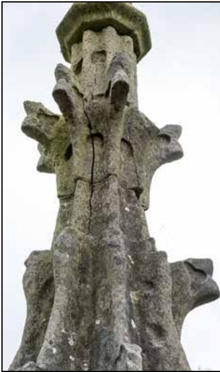
Severe cracks on the top of the pinnacle
