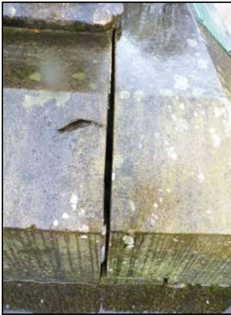
Examples of the poor state of the pinnacle
