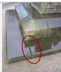
C: Open joints in bases stage of plinth allowing water ingress to base. Frost action can lead to the expansion of this joint and destabilisation of foundations if left as is. Open joints require physically closing if possible and pointing up.
